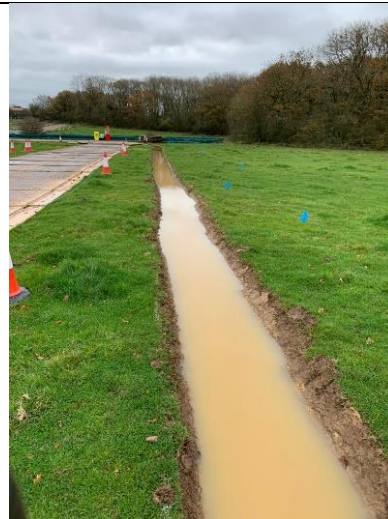
Above left: Drainage ditch during works acts to channel water from topsoil layer
