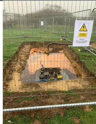
Above left: Sump collecting water from ditch network
