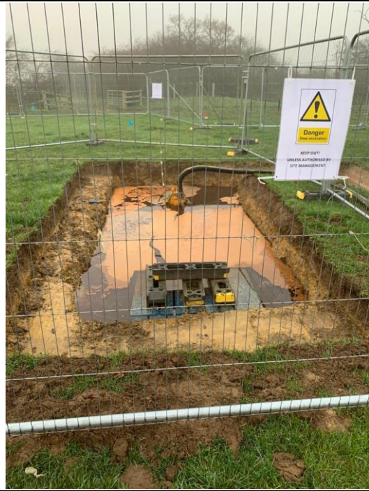
Above: Silt laden sump being pumped out – pipe leads to silt treatment system off photo to right
