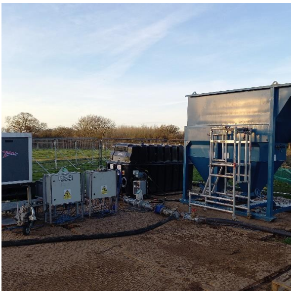
Above: Taytech silt management and monitoring system
