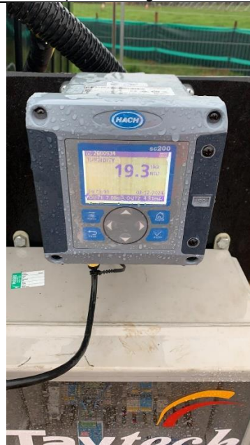
Above: Silt level monitoring device
