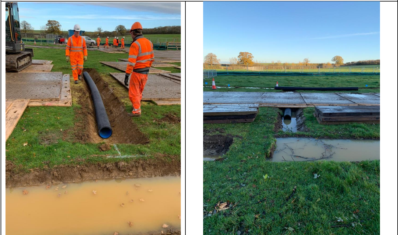
Above: Pipes laid underneath haul route to allow movement of water from central channels to sumps
