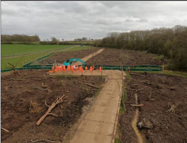
Above: Panoramic view of the receptor site showing workforce mid photo, with fallen deadwood and drainage ditches in foreground
